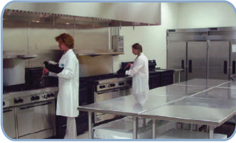
commercial test kitchen
